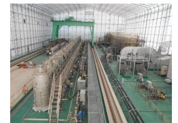
(High-performance multi-nuclide removal equipment)
