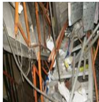
Debris on access path
