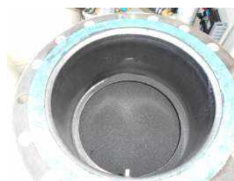
吸着槽1(活性炭上面)②
