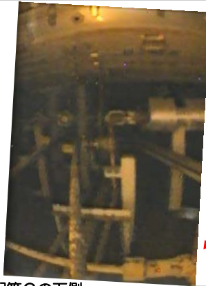
主蒸気配管Cの下側
