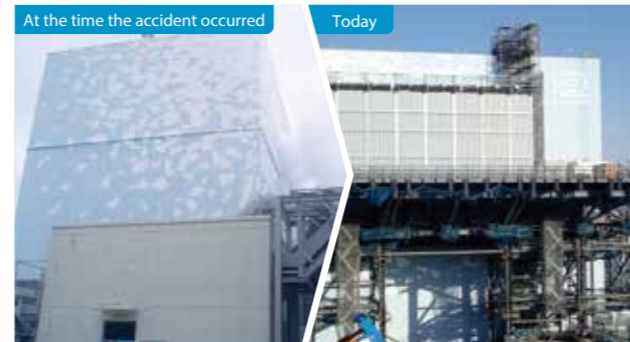
Preparations are underway to install a gantry on the south side prior to fuel removal.
