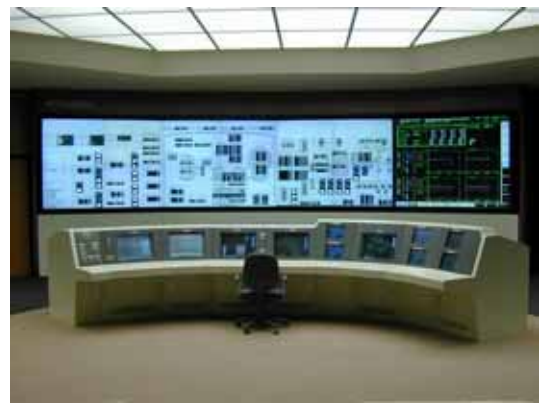
Fig. 12-2 Main Control Panel of the Latest PWR -proto type-
