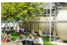
▲ Johkasou in hospital
