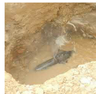
▲Identified water leakage point
