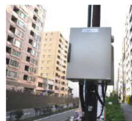
▲Flood Warning Unit for Road
