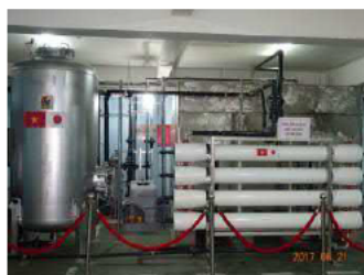
▲ Water purification equipment
