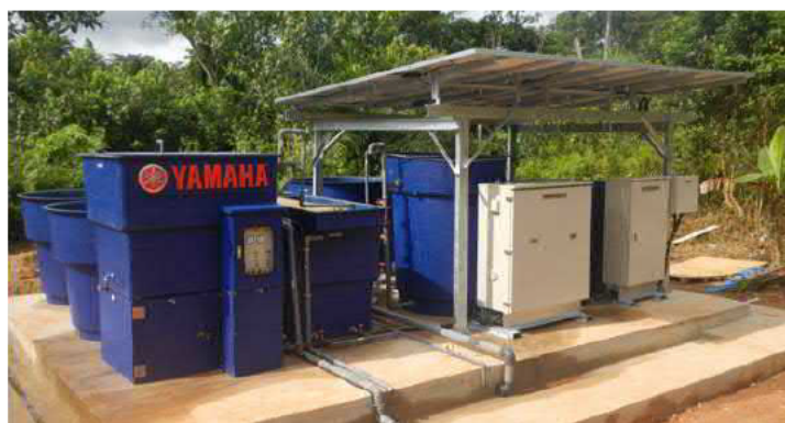
▲Yamaha Clean Water Supply System
