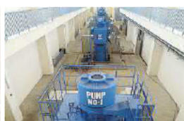
▲ Dual purpose pump station
