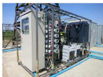
▲Water treatment system introduced to Myanmar
