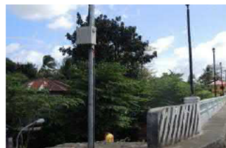
▲Installed Alarm Unit (City of Iloilo)
