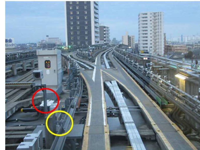
Turnout (Point Machine(Red) and movable guide(Yellow))
