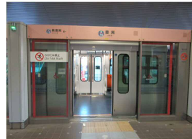
Example of platform screen door (Yurikamome : Toyosu Sta.)
