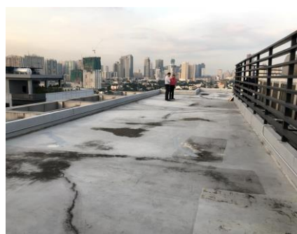
▲ Cracks on a building roof (Philippines)
