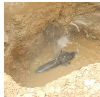
▲ Identified water leakage point
