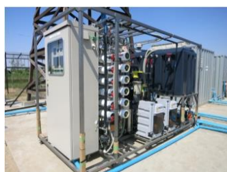
▲ Water treatment system introduced to Myanmar
