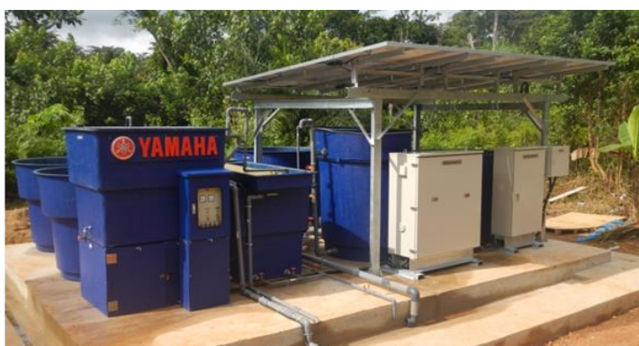
▲ Yamaha Clean Water Supply System
