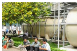
▲ Johkasou in hospital
