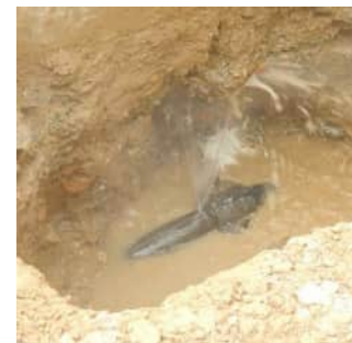
▲ Identified water leakage point
