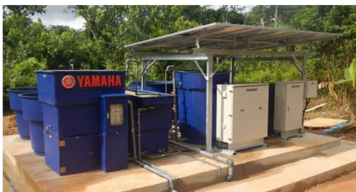
▲ Yamaha Clean Water Supply System
