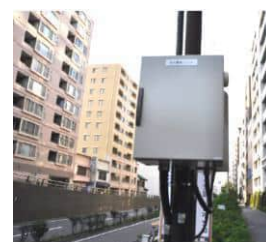
▲Flood Warning Unit for Road
