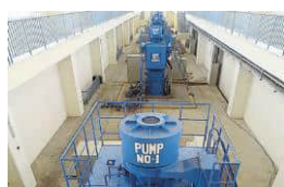
▲ Dual purpose pump station
