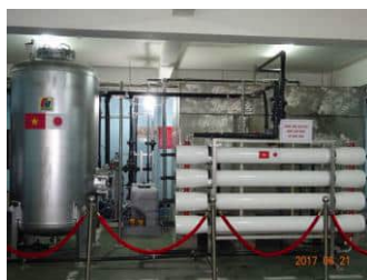
▲ Water purification equipment
