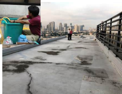
▲ Cracks on a building roof (Philippines)
