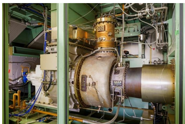
Figure 3 2MW-class gas turbine (liquid ammonia combustion) (Source: IHI)
