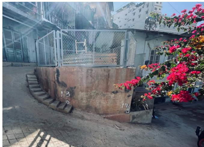
▲ Completion of landslide countermeasure works by well and drilling in Dalat city
