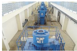
▲ Dual purpose pump station
