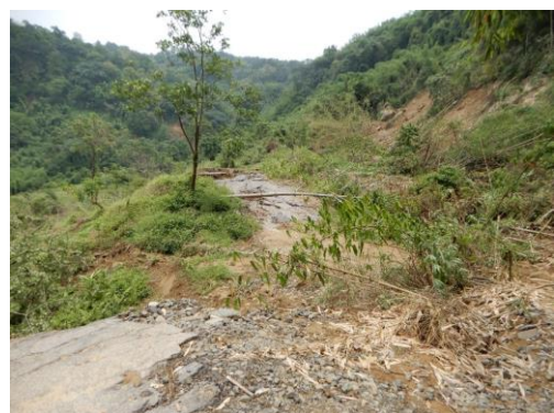
▲ View of the mountain road where the slope collapsed due to heavy rain
