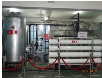
▲ Water purification equipment
