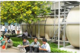
▲ Johkasou in hospital
