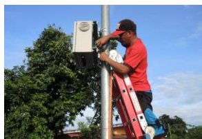
▲Installation of Alarm Unit (City of Iloilo)
