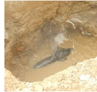
▲ Identified water leakage point
