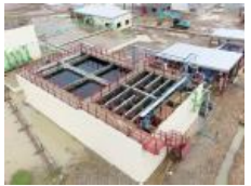
▲ Water purification plant built in Zone A, industrial park in the Thilawa SEZ
