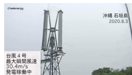
▲ Power generation experience at a maximum instantaneous wind speed of 30.4m/s.
