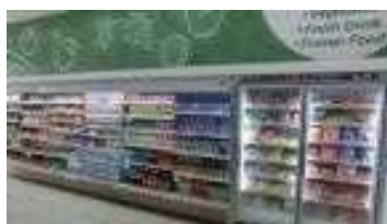
Energy saving at convenience stores, Panasonic, Indonesia
