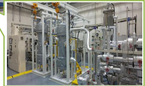
Methanation test equipment of 12.5 Nm 3 /h class
