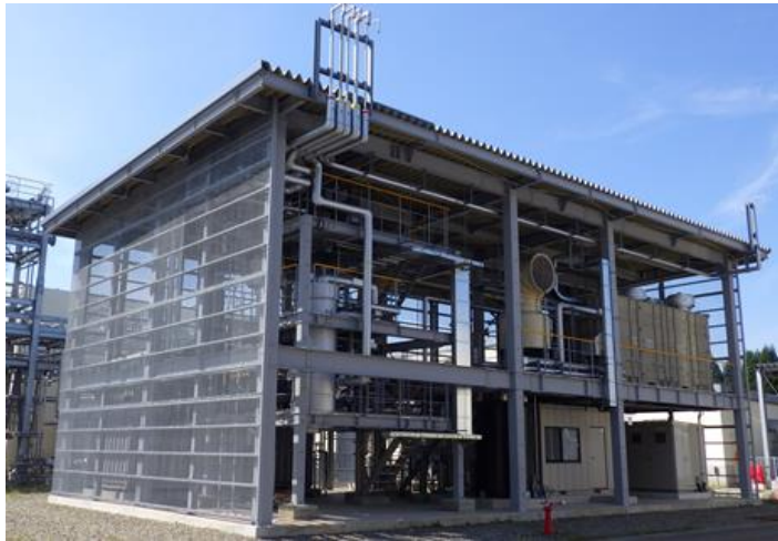
8 Nm 3 /h class methanation test equipment
