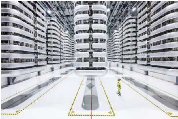
HVDC Light® Valve Hall
