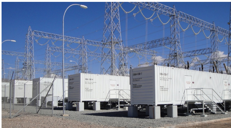
Photo of a storage project in Chile using NEC's GSS® Grid Storage Solution which will be used in the Ørsted storage project
