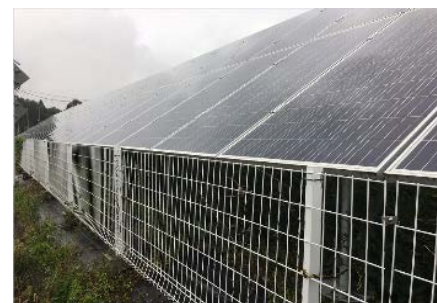
(不適切な柵塀設置の事例)
