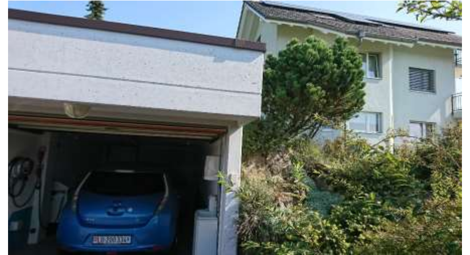
EVTEC installation @ private home in Switzerland
