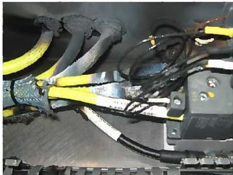
Figure 13-2: Example of overheated connections
