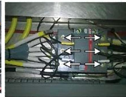
Figure 13-5: Screws in the primary terminals
