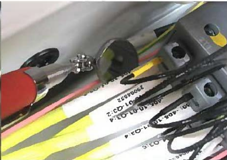
Figure 13-4: Examine the underside of the connections with a dentist mirror
